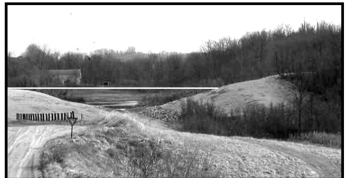
Photograph of dam breach from downstream. White line shows former dam crest.
