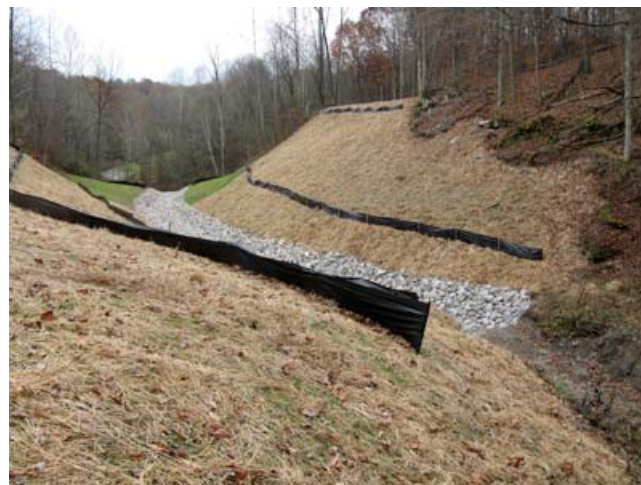
(Far left) A stream subsidence capture directs water into a deep mine opening resulting in AMD production downstream; (left) rock lined channels carry the restored stream and surface waters after construction.
